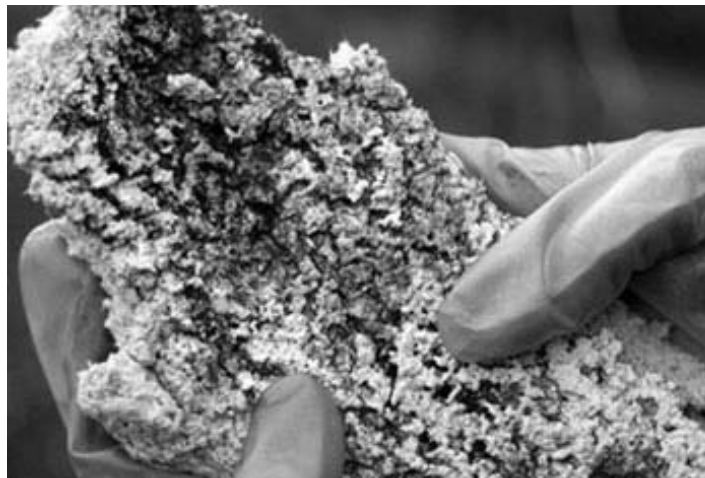
Mold growing on a piece of ceiling tile. If mold is a problem in your community association, clean up the mold and get rid of the excess water or moisture. (Photo courtesy of Environmental Protection Agency.)
