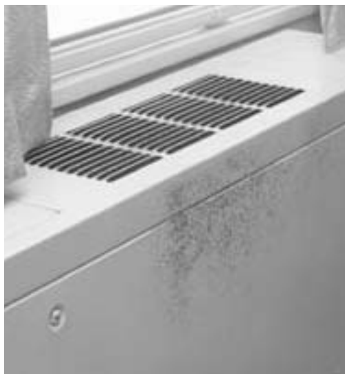
Mold growing on the surface of a unit ventilator. Moisture control is the key to mold control. If items are kept dry, mold does not grow. (Photo courtesy of Environmental Protection Agency.)
